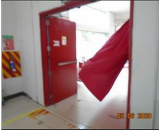
Photo of fire safety equipment Fire Door.JPG
